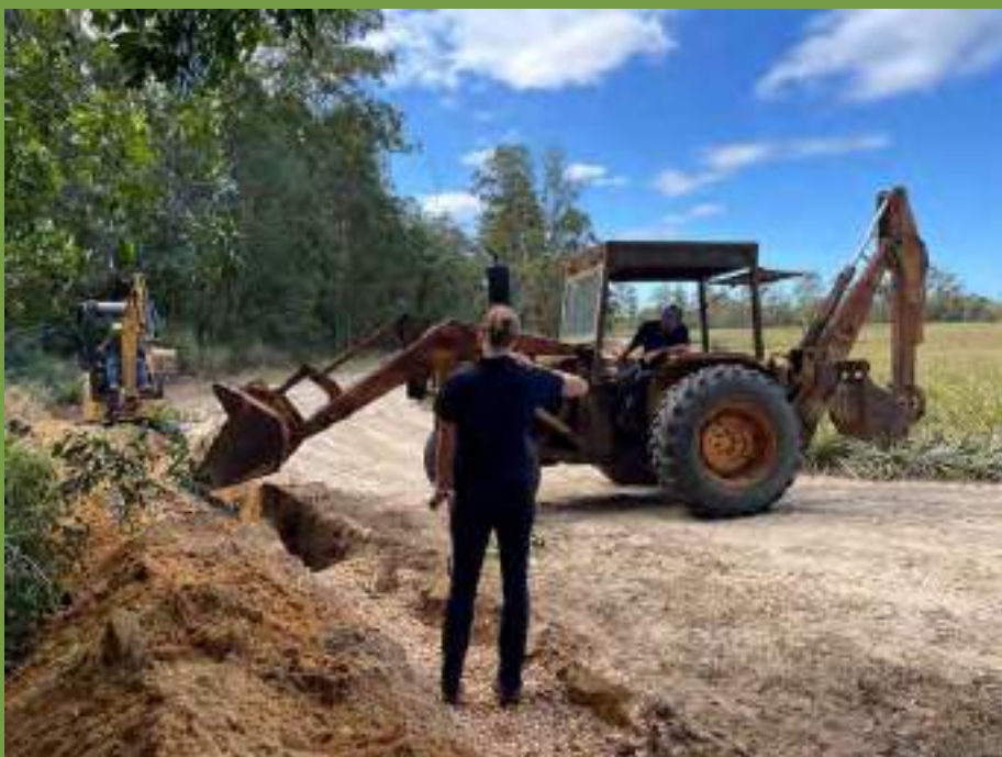
Photocaption by S.I-Brown: Woodchips are filled into a newly excavated trench to construct a denitrification bioreactor removing nitrate-nitrogen in shallow ground water before it enters the surrounding environment at the perimeter of a pineapple farm in the Glasshouse Mountains, Australia.
