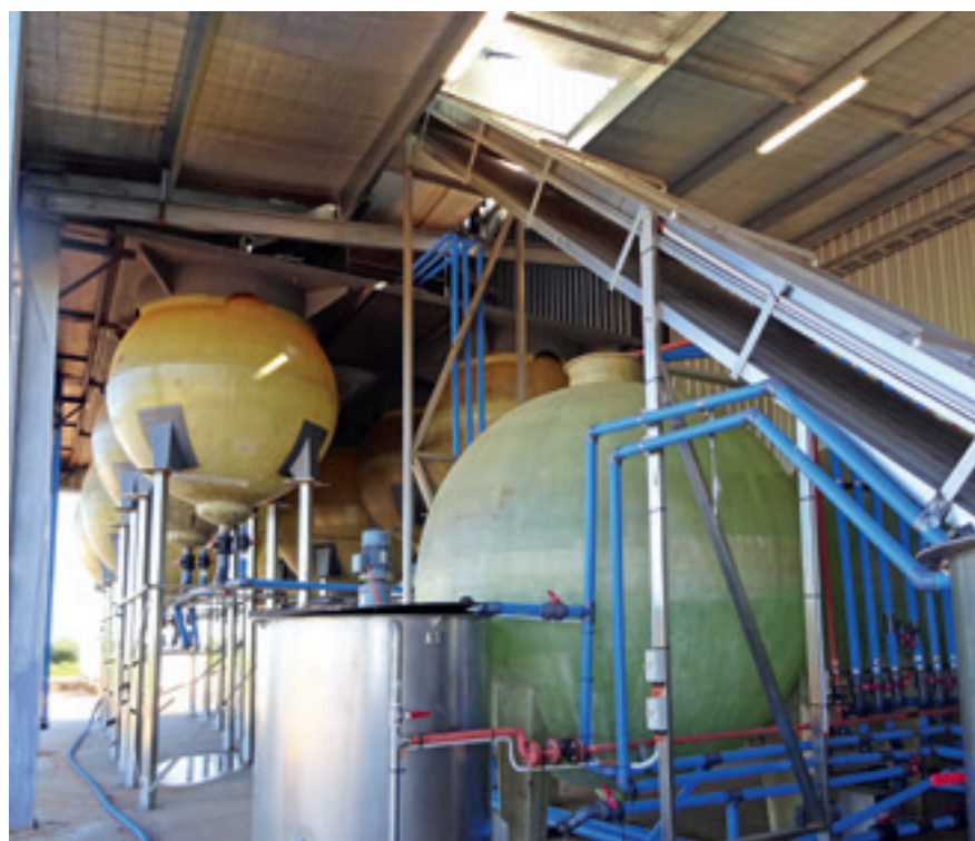
› Bulk storage of table olives going through the curing process, at Treetops Plantation, New South Wales, Australia.
